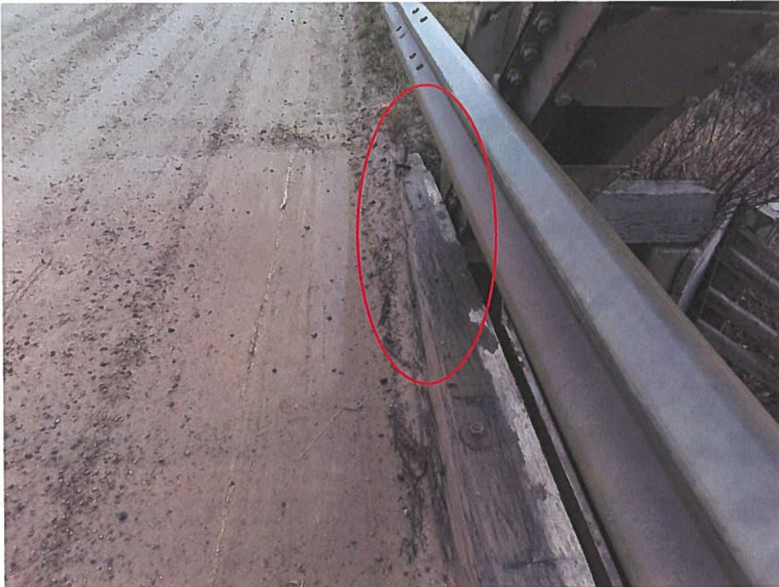
Damaged wheel guard at n/e
