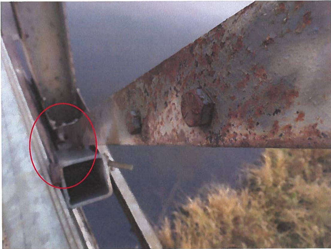
U2L3W- broken bolt connection
