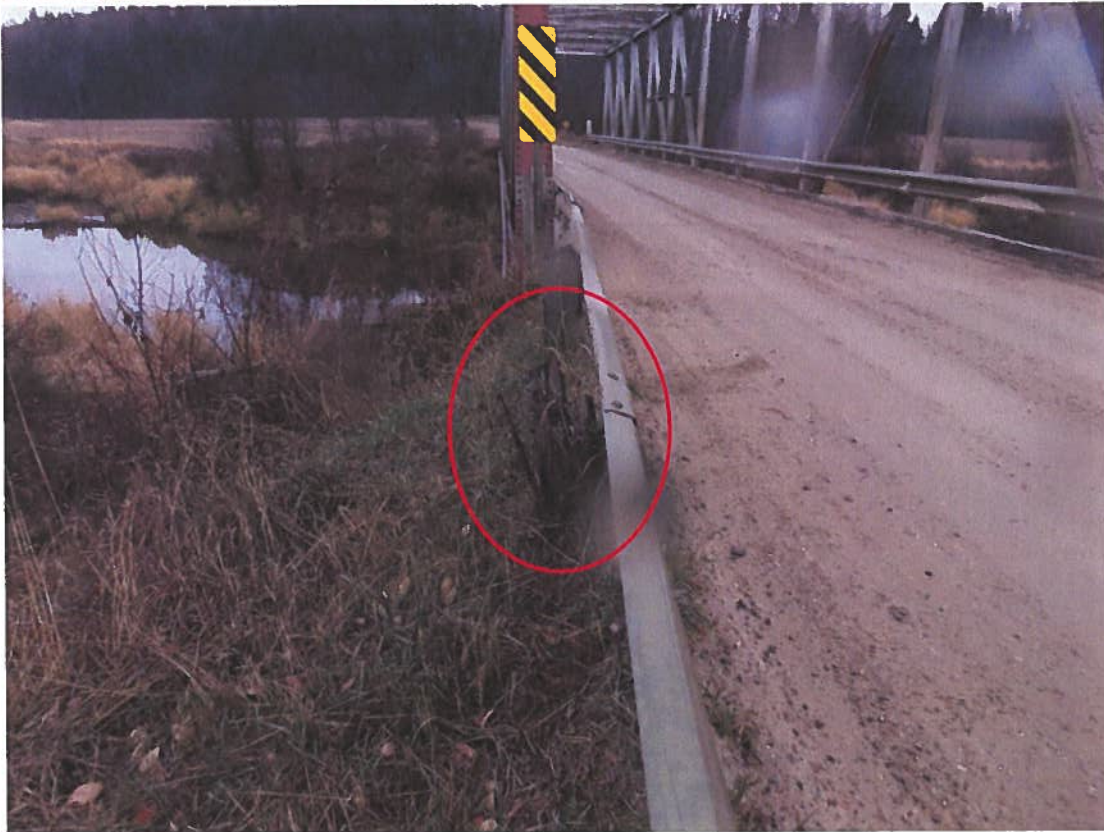
Broken guardrail post at n/e
